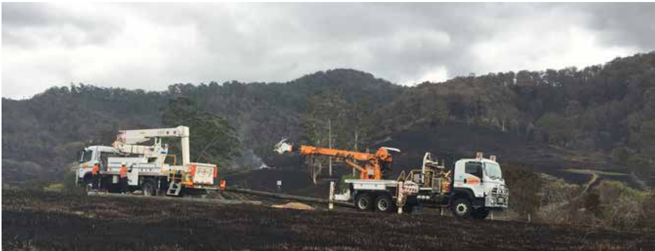
In February 2017, Essential Energy field employees worked to restore power following the devastation of the Pappinbarra and Sir Ivan bushfires.
